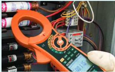
Built-in non-contact Voltage detector with LED alert
