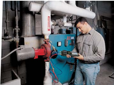
Hydronic Manometer measuring the pressure rise across a pump
