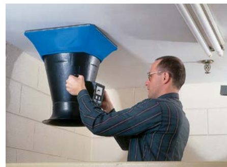
Balometer® hood measuring a restroom exhaust
